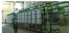
Ultra Filtration System
